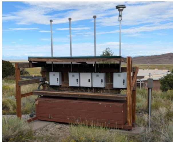
Figure 3. Photo of the GRSA stand showing disrepair.
