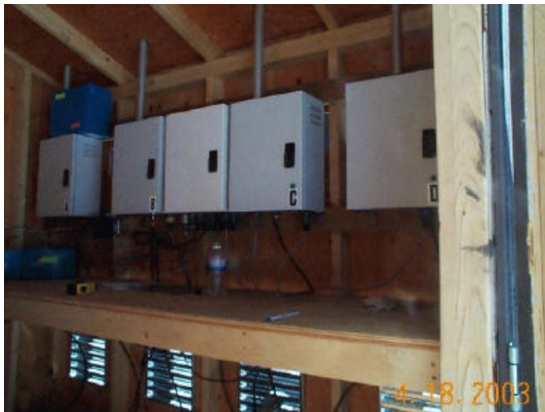
Figure 1-2. Photo of the IMPROVE aerosol sampling modules inside a shelter.
