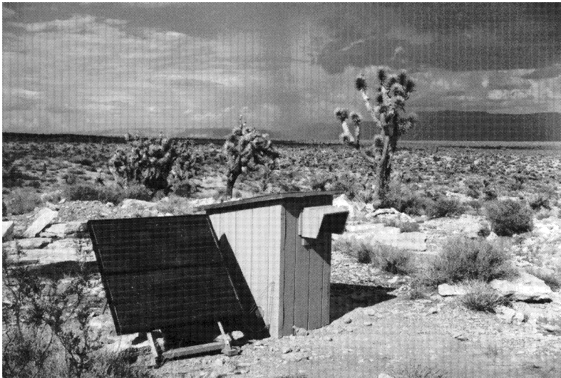
Free-standing Solar Array
